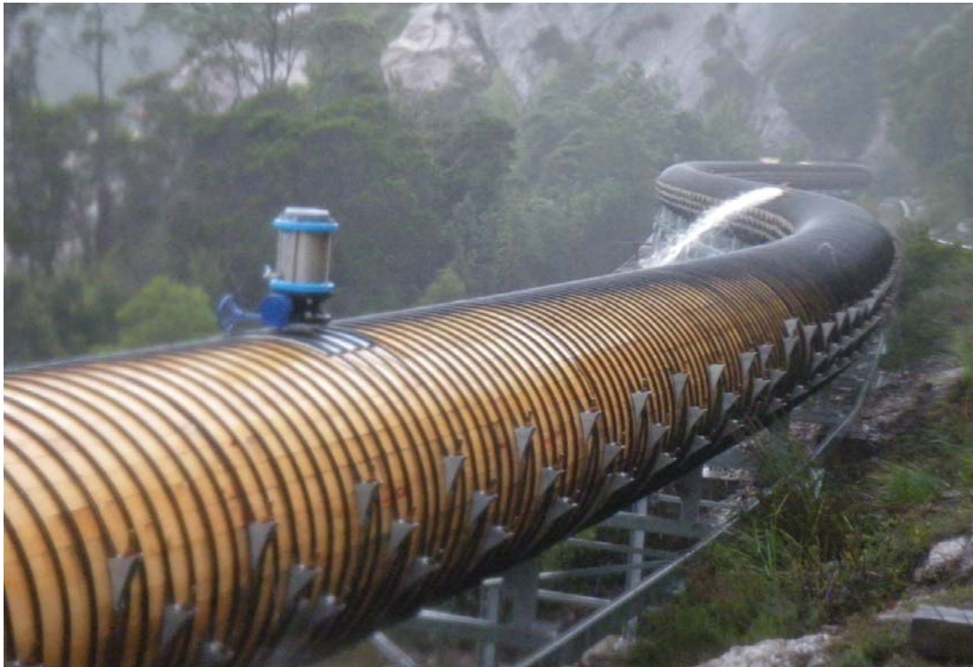
Pic 1: The new 1200mm Alaskan Yellow Cedar Woodstave Pipeline at Mt Margaret, Tasmania
